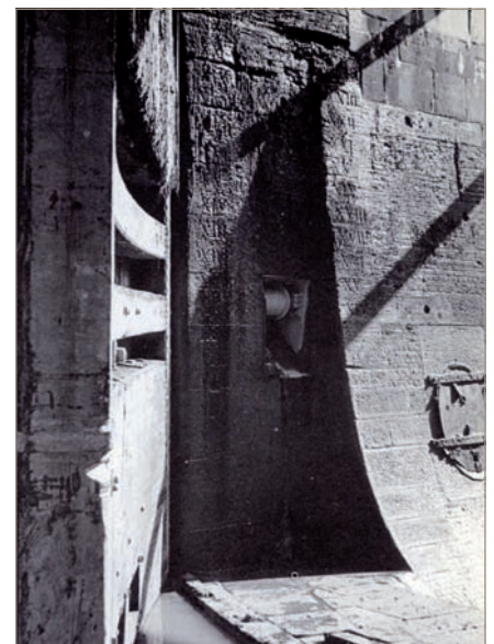
Fig. 10. Entrance lock drained down for reconstruction in 1957. Bomb damage had allowed water to flow under the lock gate platforms (Museum of London in Docklands collection)
